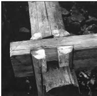
Figure 11. Corner-joint (of head beams and post) in an old house in Mi(d)vágur, photoed by Sverri Dahl 1952 when the house was under repair.
