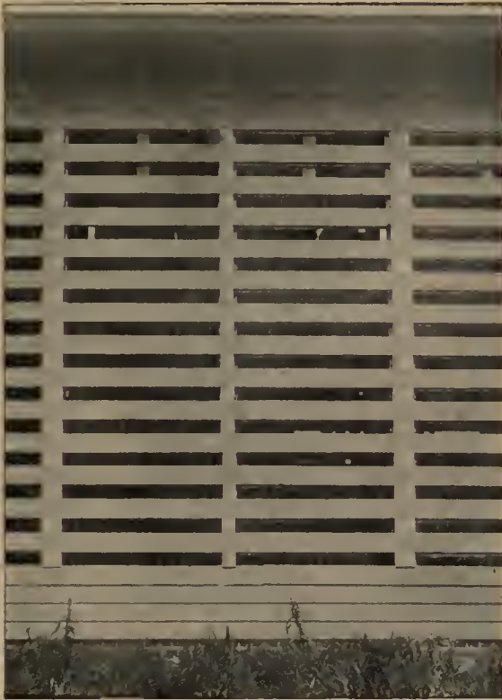
UNIQUE VENTILATION SYSTEM OF THE SHED OF THE SCHMIDT & BUNGE LUMBER COMPANY, AVOCA, IOWA. SIX-INCH STRIPS ARE NAILED TO THE SIDE OF THE BUILDING, WITH SIX-INCH SPACES BETWEEN THEM. INSIDE THERE ARE FRAMES FOUR FEET WIDE, ON WHICH THERE ARE NAILED CORRESPONDING SLATS. THESE FRAMES ARE MOVABLE SO THAT BY RAISING THEM SIX INCHES THE VENTILATION IS SHUT OFF, THE SIDE PRESENTING A SOLID APPEARANCE.
