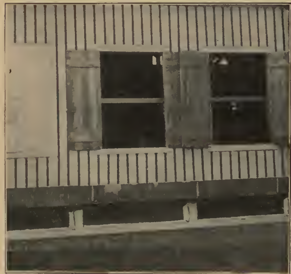
VENTILATING SYSTEM OF THE CRANE-JOHNSON SHED, COOPERSTOWN, N. D. AT THE BOTTOM OF THE WALLS ARE DROP DOORS, FOURTEEN INCHES WIDE, ALSO DOORS OPENING IN THE REAR OF THE PILES. THE FOUNDATIONS FOR THE PILES BEING FOURTEEN INCHES HIGH, THUS PROVIDING FOR A SUPPLY OF AIR BOTH UNDER AND THROUGH THE LUMBER.
