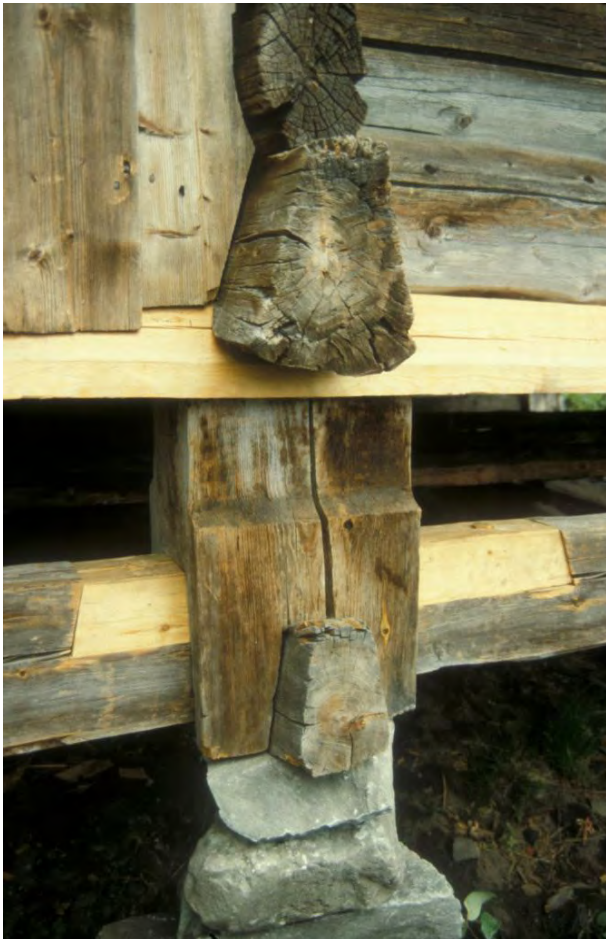
Figure 5.10 Repairing a medieval storehouse in Tokke, Norway. The structure is repaired in situ without dismantling. New, well-seasoned wood is jointed in.
