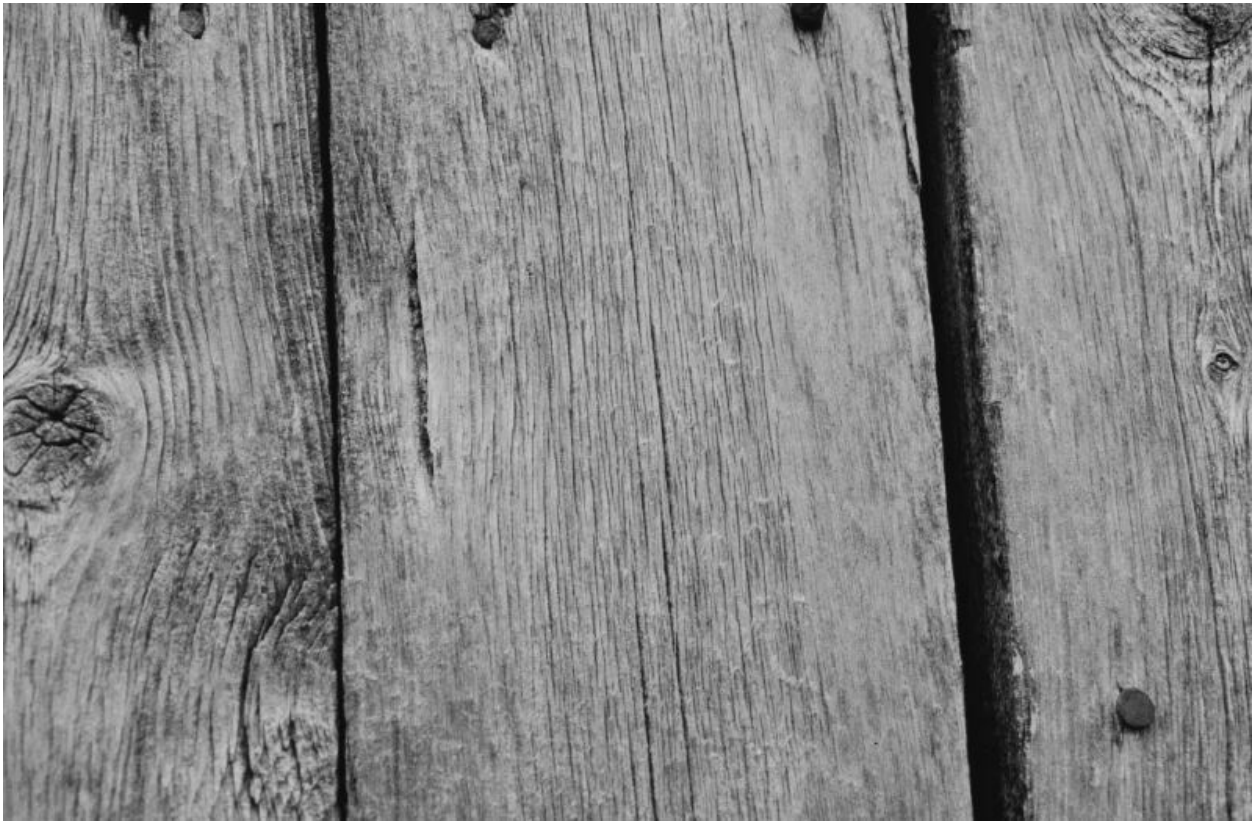
Figure 8.5 External boarding of aspen ( Populus tremula ), about 80 years old. This external boarding has never been treated with paint or coating. It is still in excellent condition, despite being on an exposed site.
