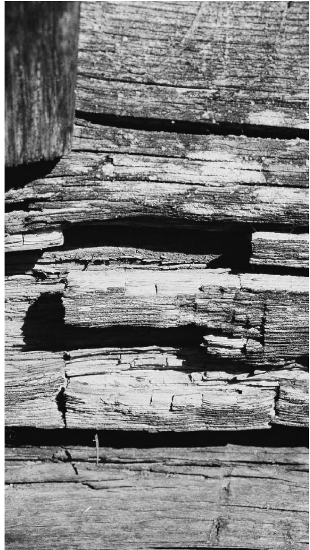
Figure 9.1 Brown rot showing typical cubical deterioration of wood.
