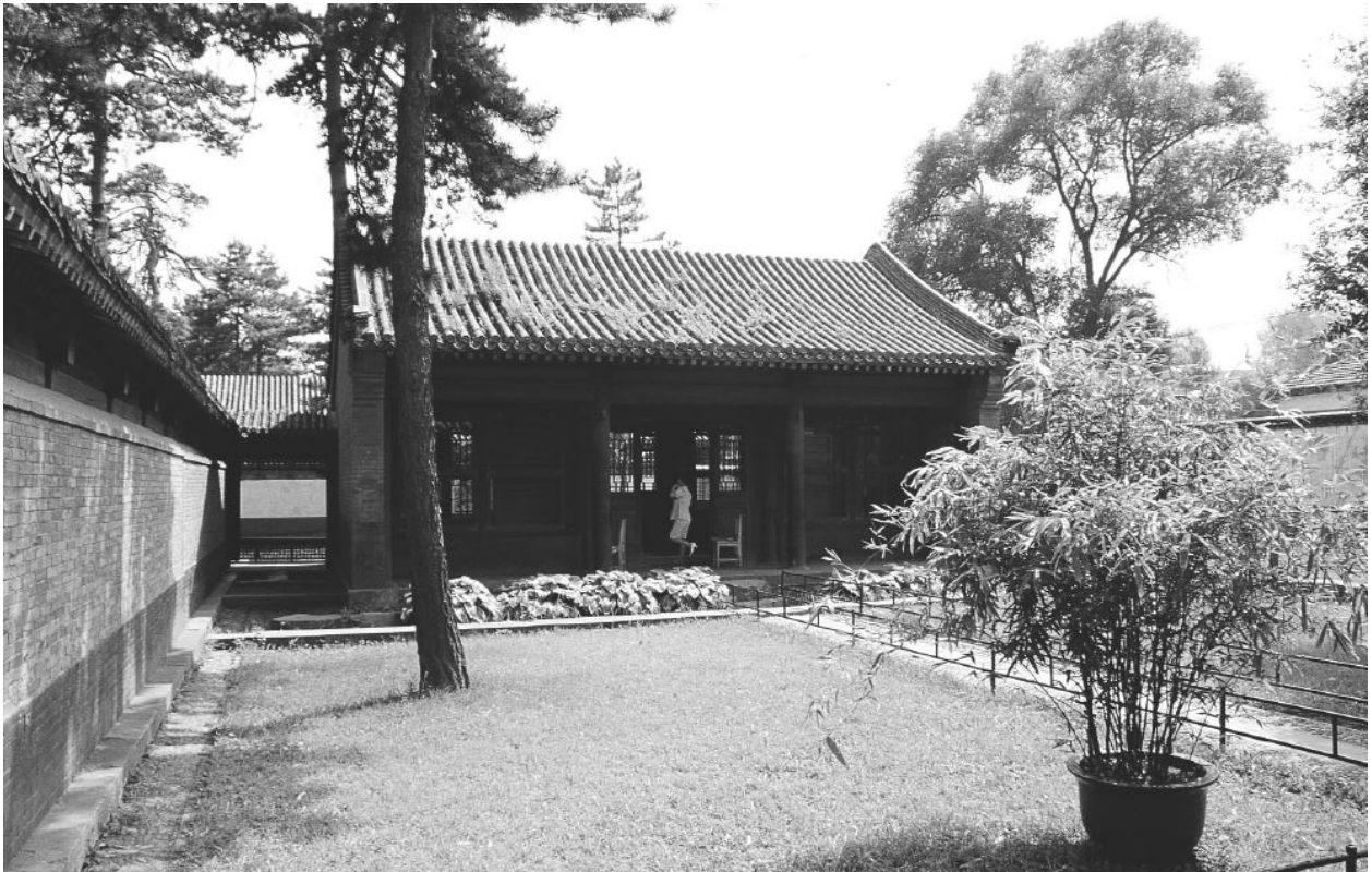
Figure 7.11 The Mountain Resort, Chengde, China, a World Heritage site. Small trees are growing on the roof of the building in the background. It is a part of the site management plan to remove growth from the roofs every three years. The removal is necessary for the long-term protection of the roof timber structure and tile roofing. The roof in this picture had been cleaned one year previously.
