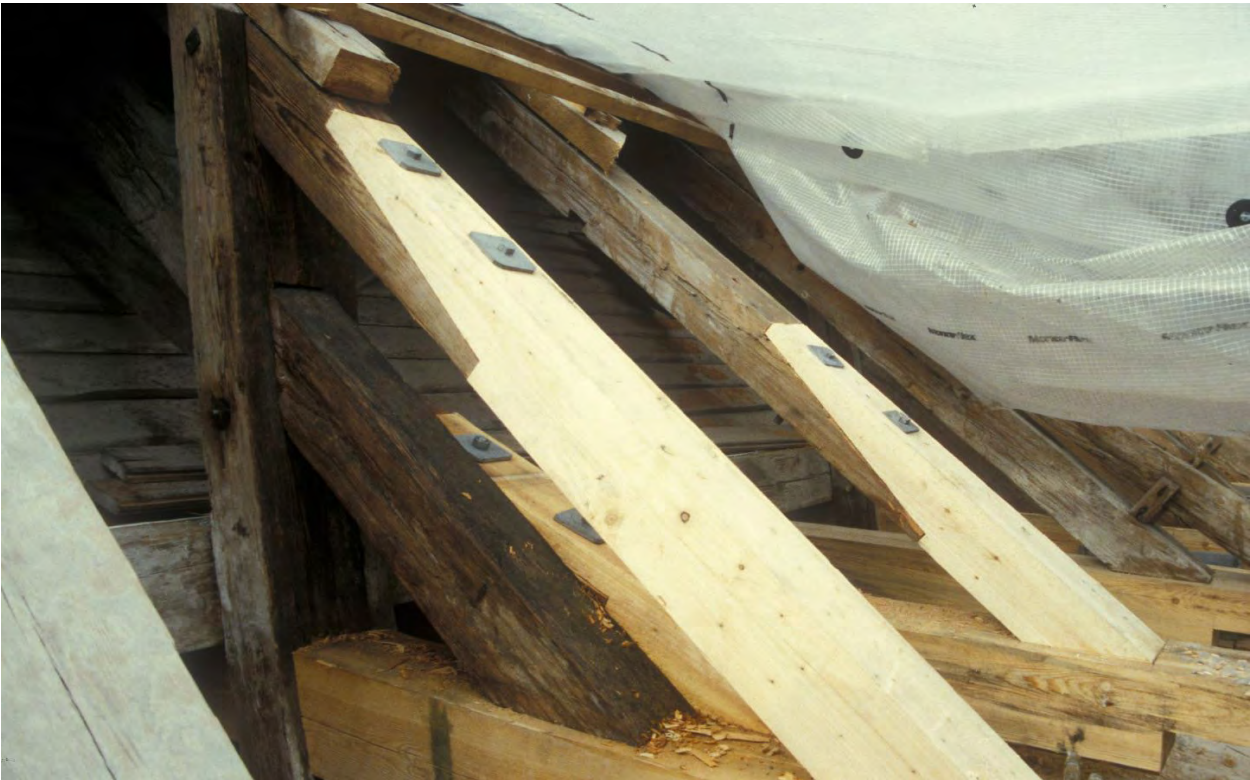
Figure 4.1 Hørsholm church outside Copenhagen, Denmark. Repair of rafters 1997. New and old timber is jointed and the joint reinforced with steel bolts and toothed-plate connectors.
