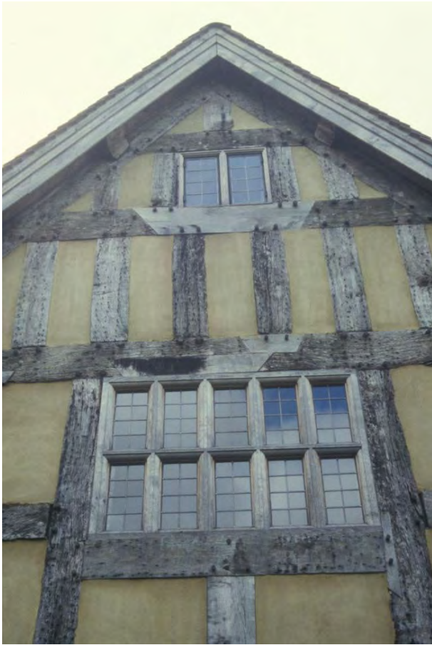
Figure 2.3 Brookgate Hall after restoration. Detail of a gable showing replaced timber in the frame. Brookgate Hall after restoration. Detail of a gable showing replaced timber in the frame.
