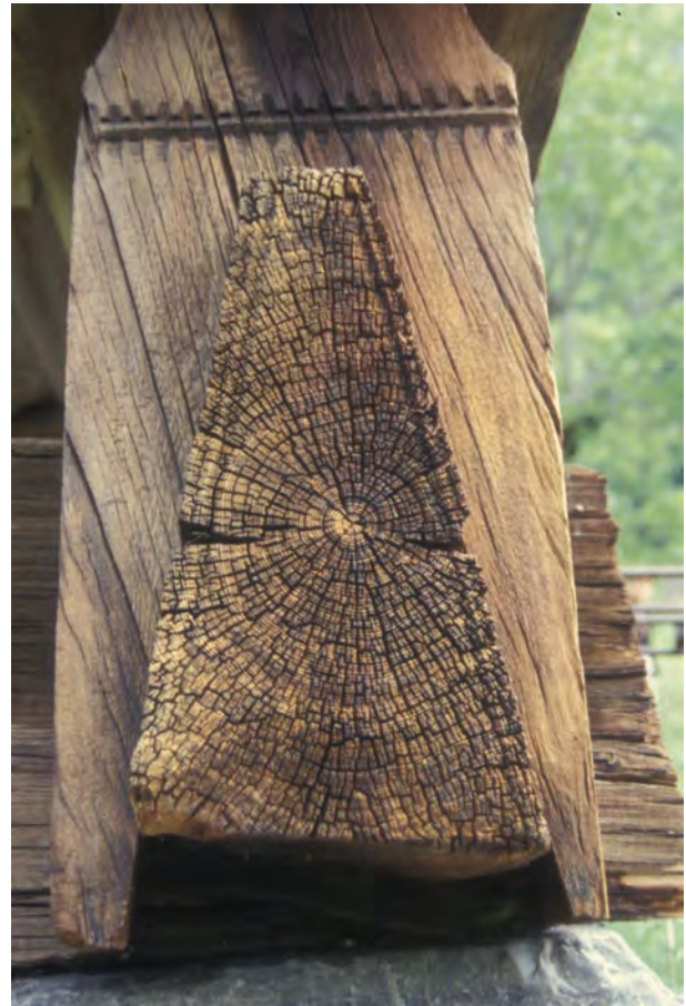
Figure 8.8 Detail of the sill-beam in a Norwegian log-structure from late eighteenth century. Note the extremely narrow width of the annual rings, and that the sapwood content is insignificant. It is very well preserved, despite exposure to the elements over two centuries.
