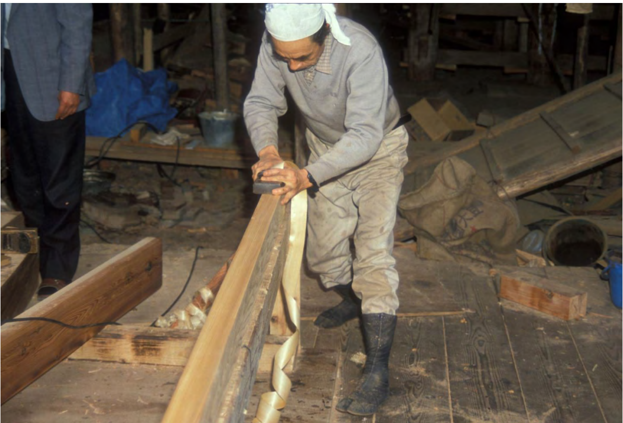
Figure 5.7 Carpenter at the repair site of the three-storied pagoda of Oyama-dera, Ibaraki, Japan in 1989. planing. The long, perfect shaving is a trademark of the excellence of Japanese carpentry work. The carpenter is pulling the plane.
