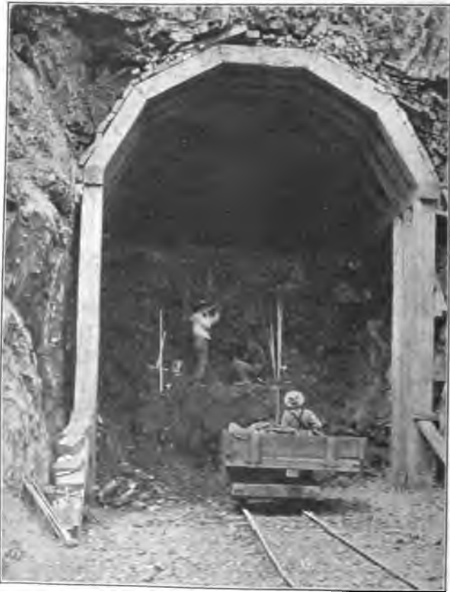
FIG. 287. Segmental timbering, used in tunnel work on the Western Pacific Railway. See Railroad Age Gazette , vol. 45, page 902, Sept. 11, 1908.
