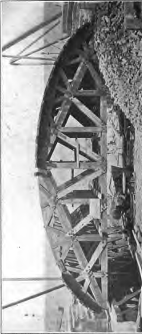
FIG. 75j. Centers for an Elliptical Arch at 138th Street, Riverside Drive, New York City.
